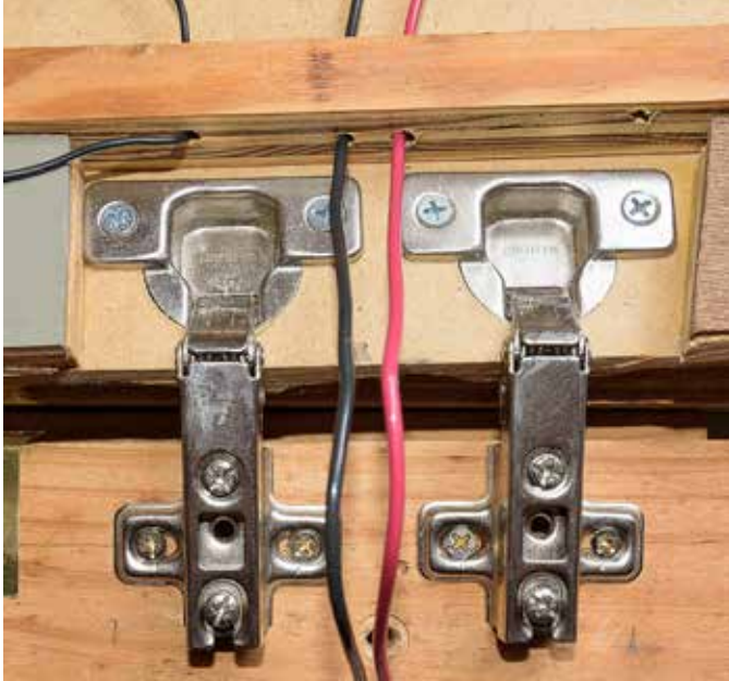
4 Final installation. This under-the-layout view shows how the hinges are attached to the lift-up section (top) and layout. Don drilled pilot holes for all of the screws before attaching the hinges to the plywood and Homasote.
