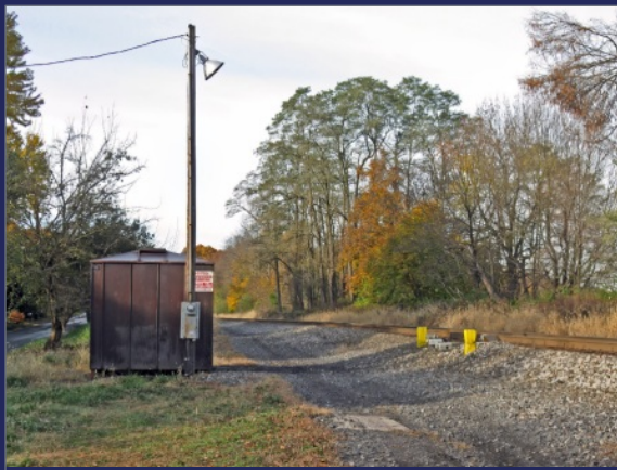
6. A defect detector installation is made up of several components mounted on the track, with the electronics housed in an adjacent equipment shed. This installation
