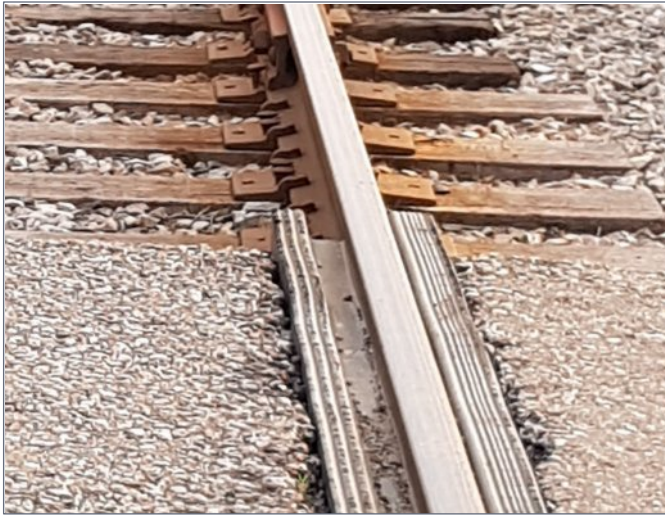
3. A closer look reveals that, while the pavement continues between the rails, there are rubber spacers between the asphalt and the rail to control the gap for the train wheel flanges.
